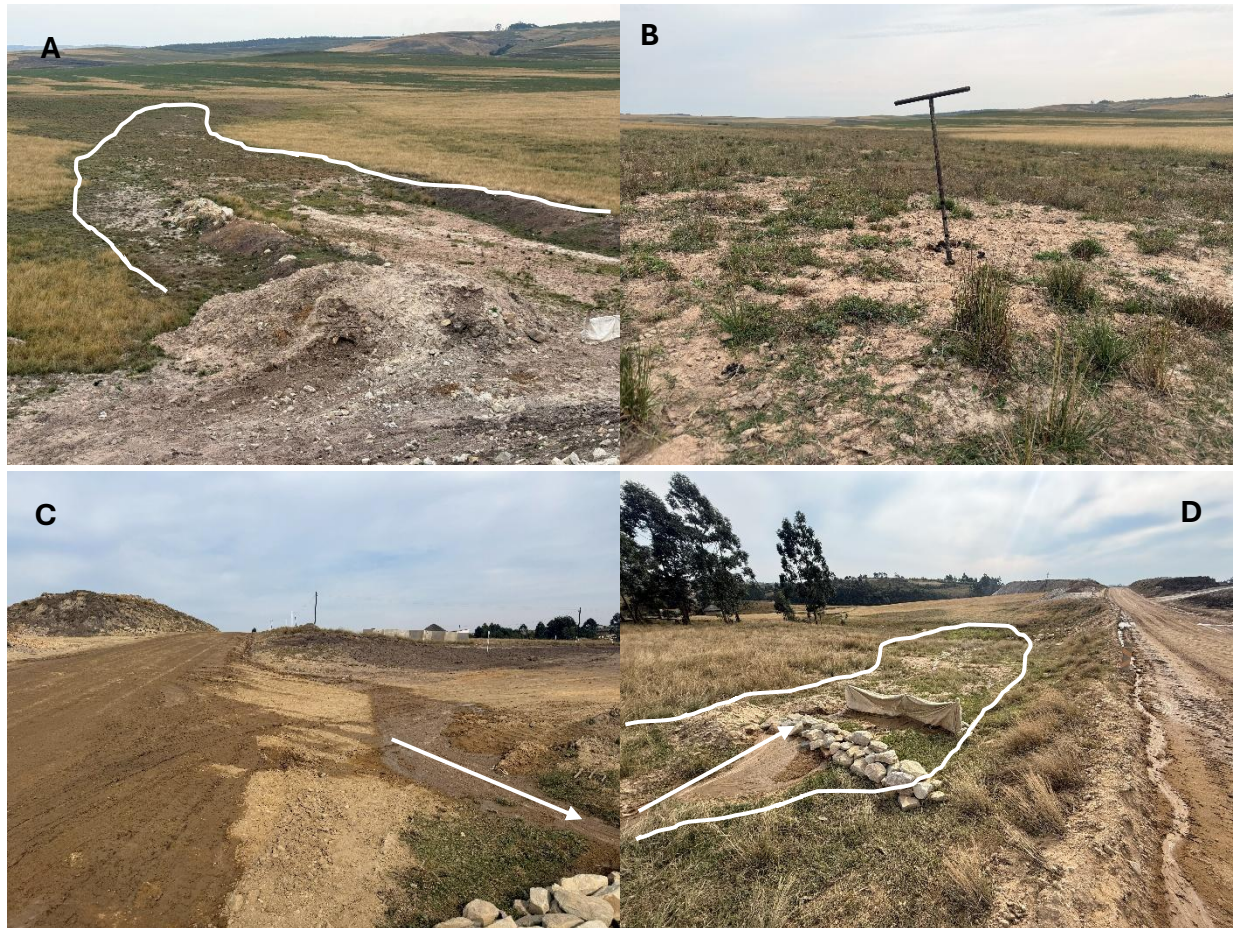
Figure 4 A) Extensive sediment deposition captured from the N2 road reserve (CI number 1), shown in Figure 3. B) Close up view of the large sediment plume shown in Figure 3, illustrating the extent to which wetland vegetation has been buried by the sedimentation. C) Source of CI number 12, with the white arrows indicating the path that water takes as it enters the wetland as shown in D). D) Impact of sediment within the wetland. Note some sediment control structures have been constructed, but they have been bypassed, or were constructed after the sedimentation event occurred. Find coordinates of all photographs in Appendix A.
